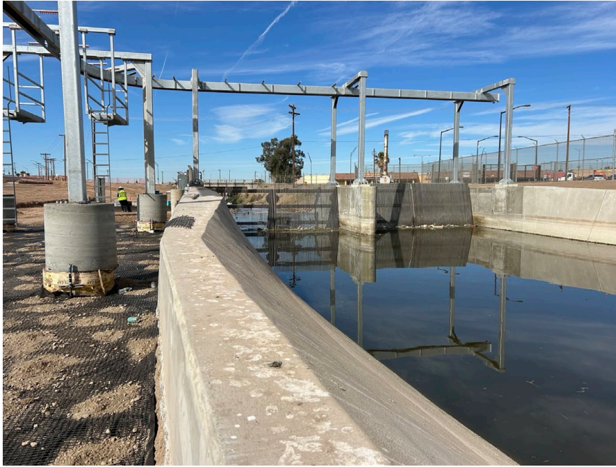
Figure 19. New River Improvement Project trash screen at the diversion structure on the New River.
