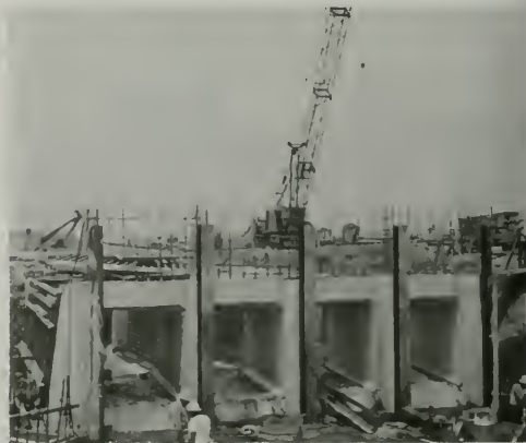
Figure 168. Sutter-Butte Canal Outlet Conduits
