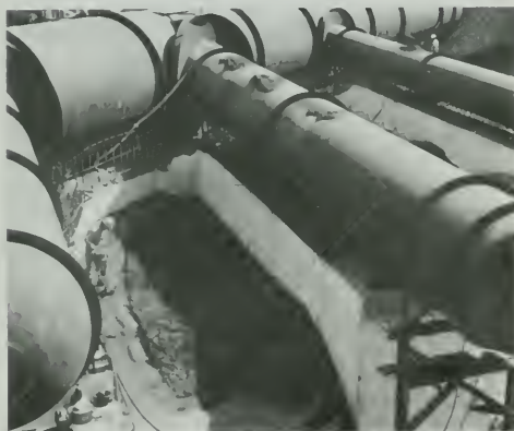
Figure 298. Outlet Works Delivery Manifold
