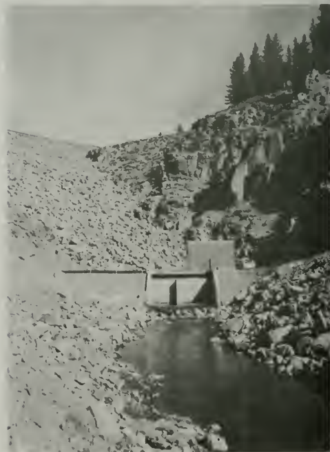
Figure 51. Control House at Dam Toe
