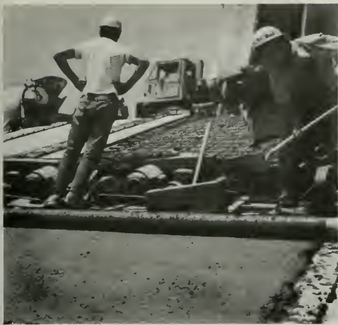
Figure 162. Closeup of Slip Form Lining Operation on Thermalito Power Canal Transition Slopes
