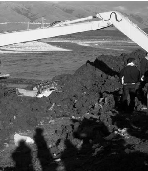
Pond A19's levee is breached. Photo by Beth Huning.
