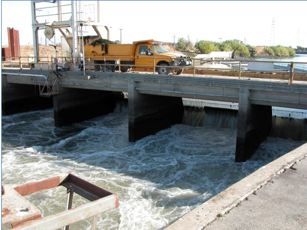
Figure A6-1.—Downstream looking perspective of the trashrack at the Bureau of Reclamation's Tracy Fish Collection Facility (Byron, CA). The image shows a significant trashrack differential, or difference in water depth upstream and downstream of the trashrack, and how such conditions create turbulent flows in the primary channel.
