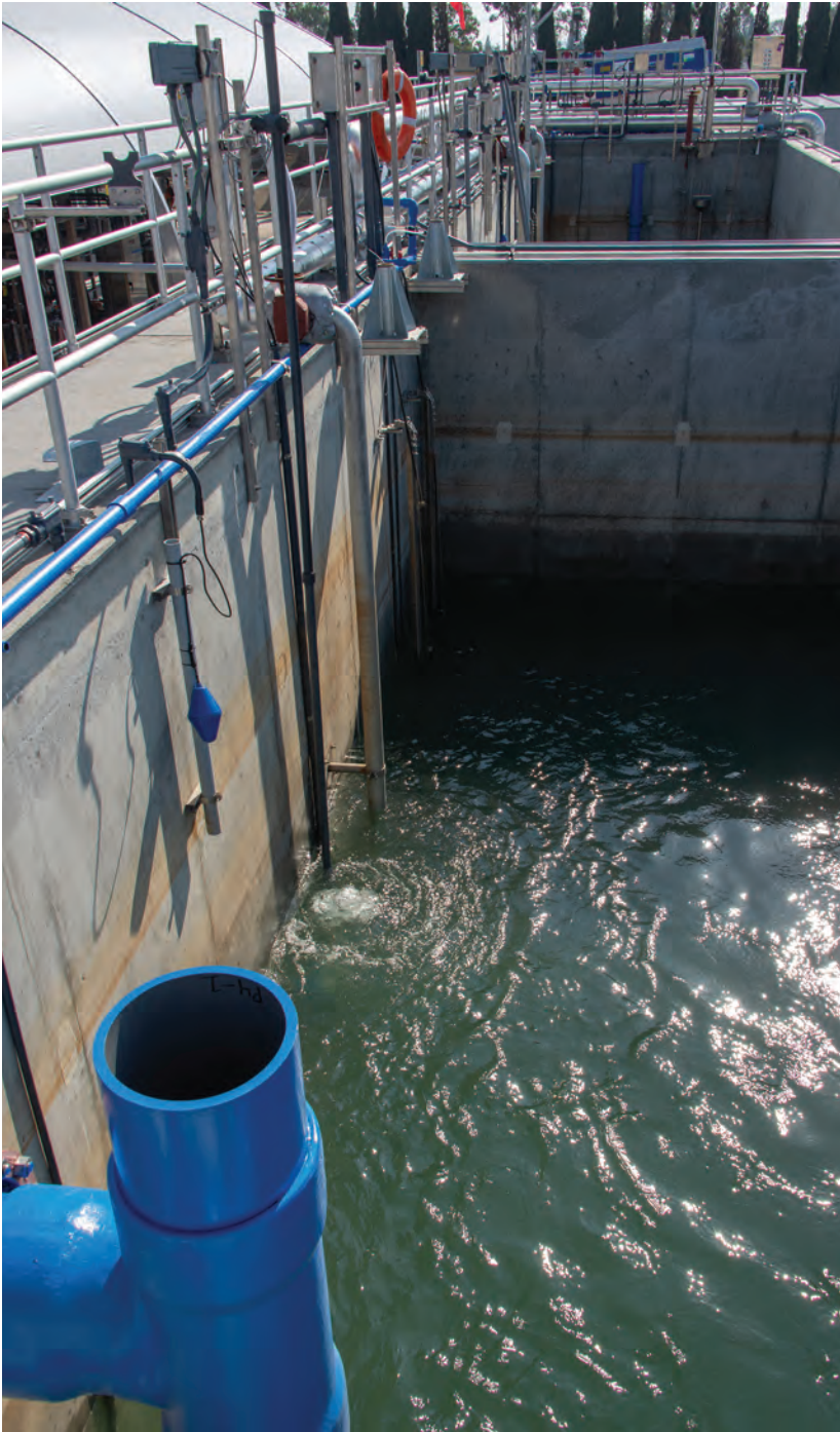
Aeration basin equipment undergoes testing at the Regional Recycled Water Advanced Purification Center in Carson.
