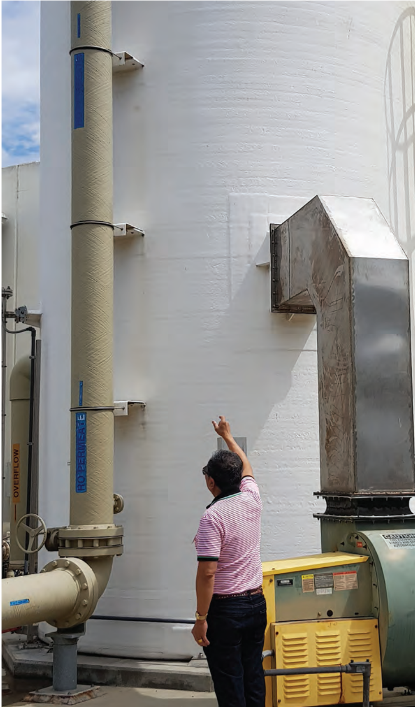
Audit staff inspects a decarbonator at Irvine Desalter Project during an audit of groundwater recovery projects funded through Metropolitan's Local Resources Program.
