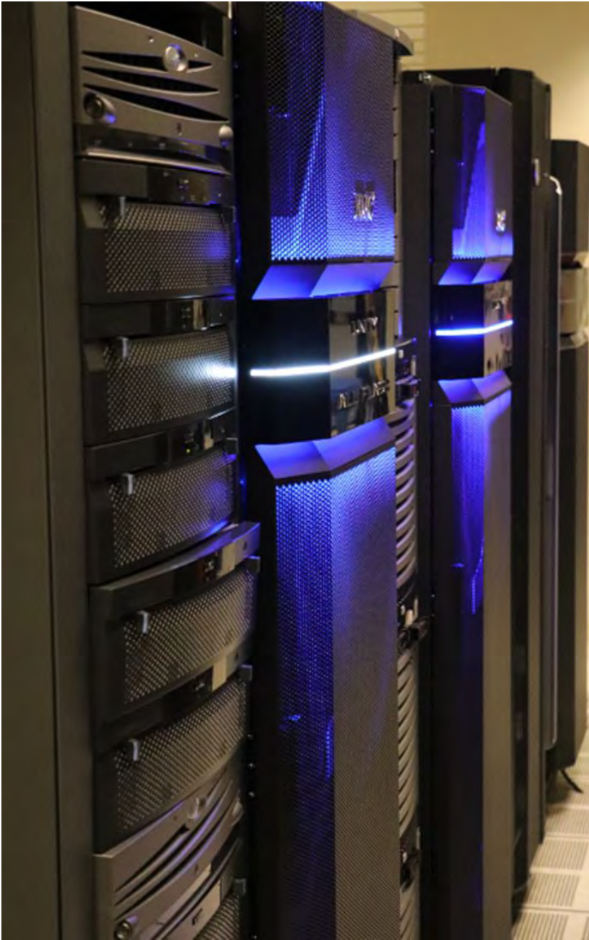
Servers located inside the data center at Metropolitan's headquarters building.
