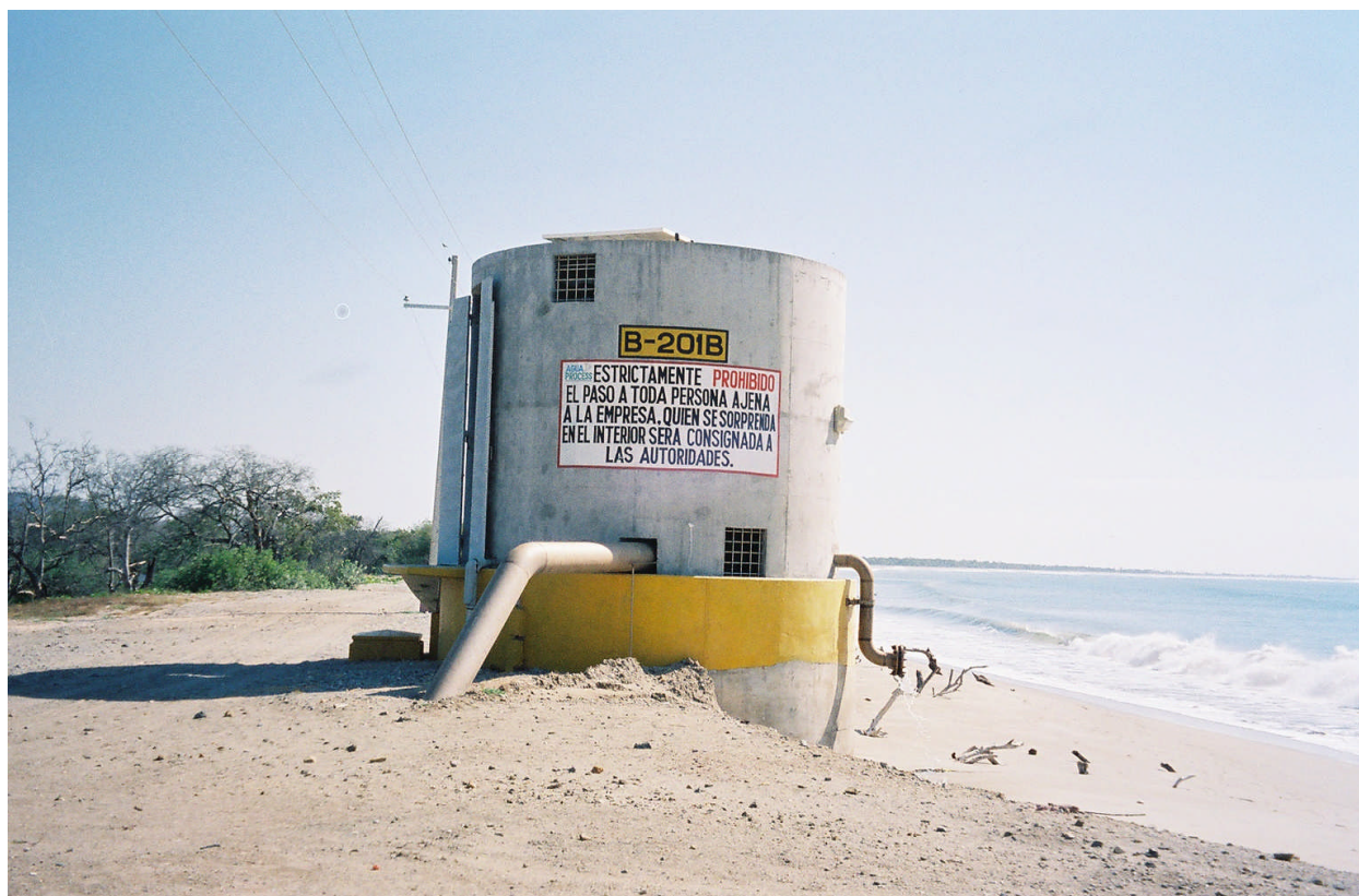
Figure 2 – 3.8 MGD Horizontal Seawater Intake Beach Well
