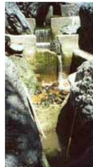
Photo 4-3 Big Chico Creek—Iron Canyon's worn concrete and collapsed floor /DWR photo
