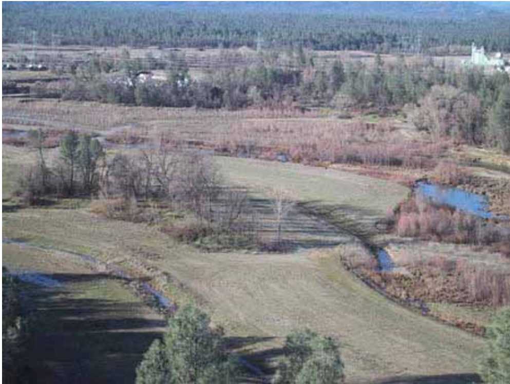
Photos 3-1 and 3-2 The Lower Clear Creek Floodway Rehabilitation overview (top photo) and the new floodplain at work
